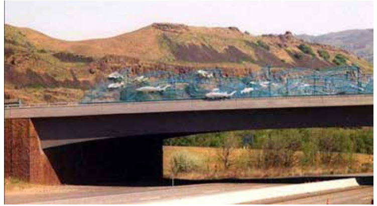
Figure 22: Example of a decorative rail reflecting a local recreational asset, in this case, salmon. Note, however, that better design consideration of background and its influence affects how well this enhancement is viewed.
