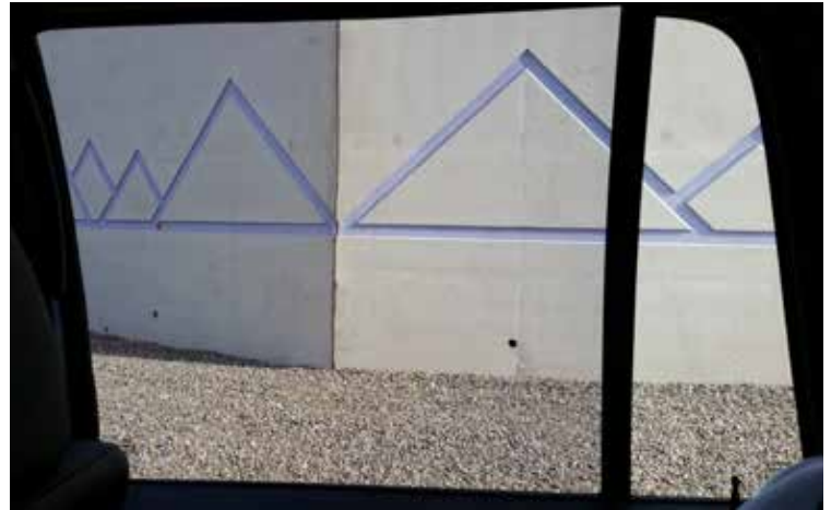
Figure 19: This simple abutment design in Phoenix is an abstract of the mountains surrounding the area
