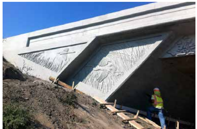
Figure 21: This concrete form liner is located along Interstate 5 near Stockton, California. Any brand element can be applied to an abutment.
