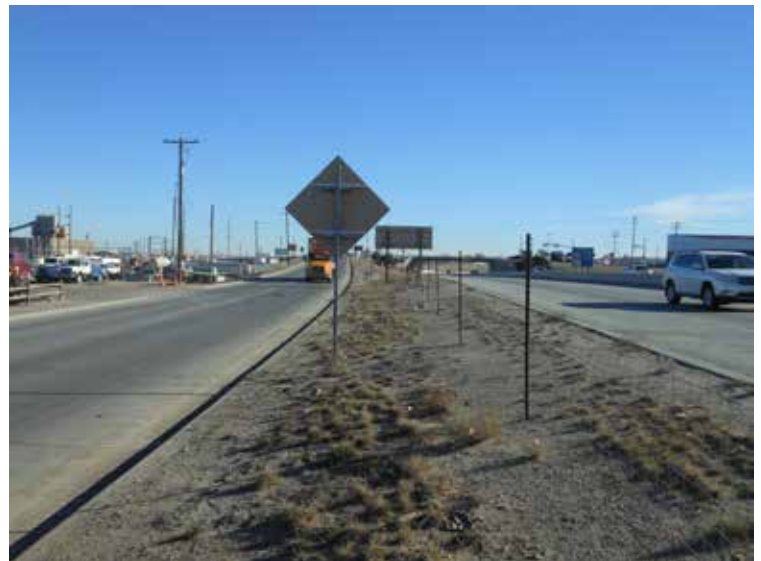
Figure 3. Example of undesirable fencing and ground cover
