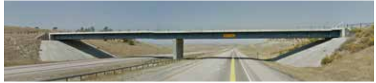
Figure 26: FHWA color 25053 (blue) girder on I-25, located approximately six miles north of Highway 259 exit in Wyoming
