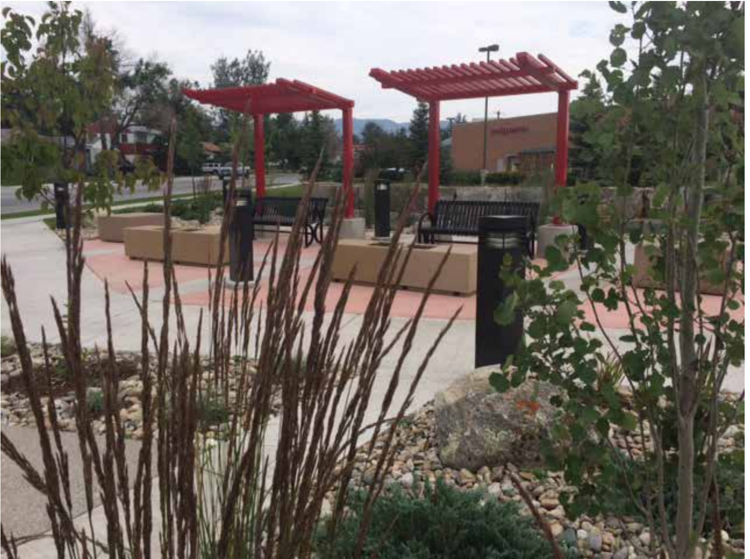
Figure 33: New pedestrian plaza at the corner of CY Avenue & Poplar Street, a City of Casper project incorporated into a WYDOT road project
