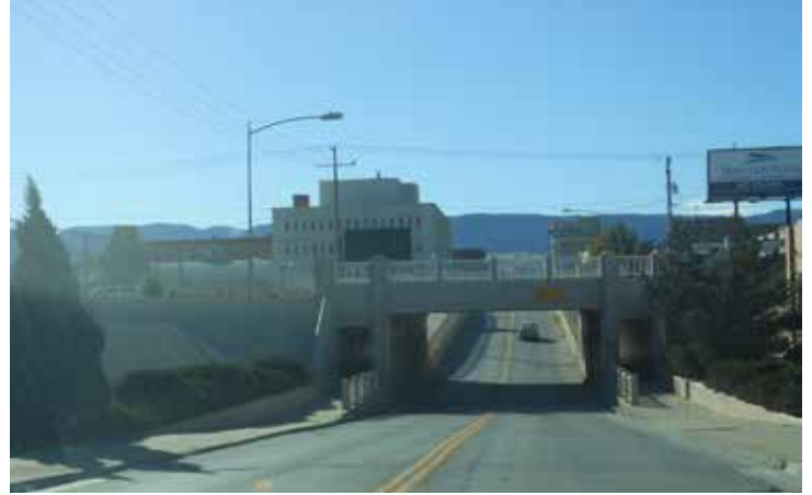
Figure 16: Example of an underpass with substandard clearance
